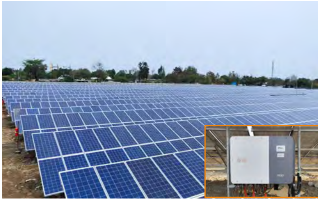
Latur Maharashtra, India 2.8MW
