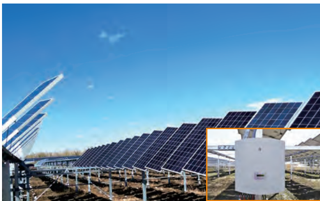
Hebei Zhangbei Agricultural-photovoltaic hybrid PV plant 50MW
