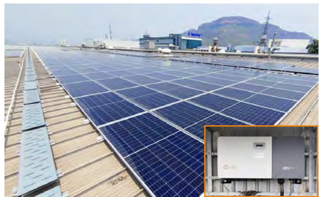
Tetra Pak Project, India 1MW
