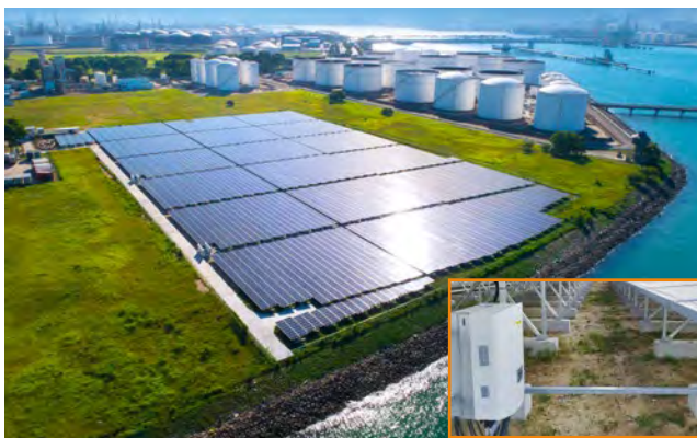
JTC Solar Farm, Singapore 5MW
